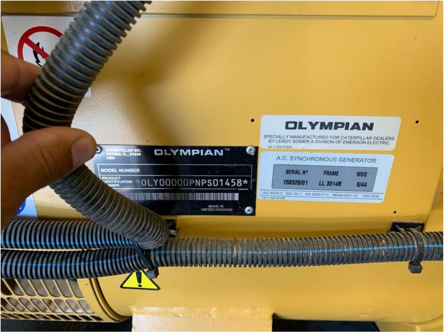
LS 14 Generator Nameplate
