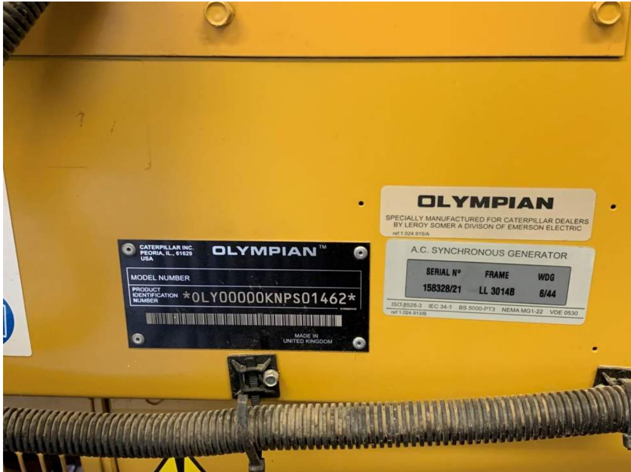
LS 13 Generator Nameplate
